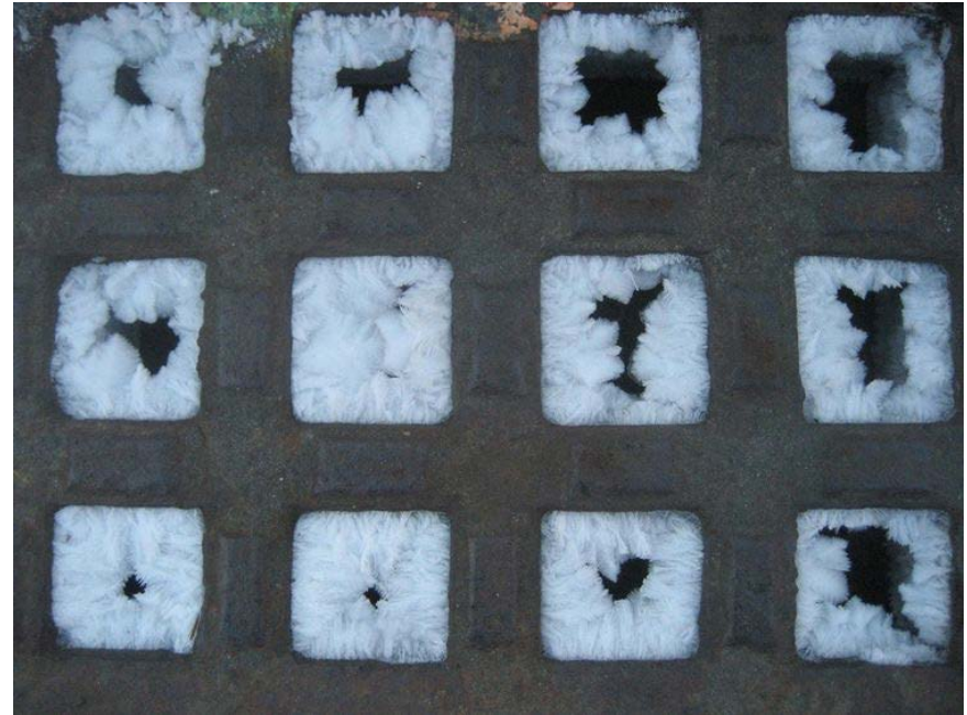
Sewer top desublimation (photo by Rob Sheridan)
